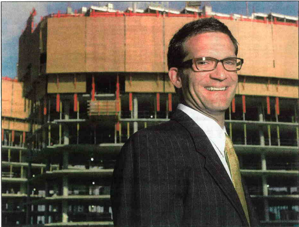
Scott Eaton of Gerding Edlen Development Co. LLC is framed by his company's $500 million Bellevue Towers as it rises across the street from the project showroom. BUSINESS JOURNAL PHOTO/DAK SCHLATTER
